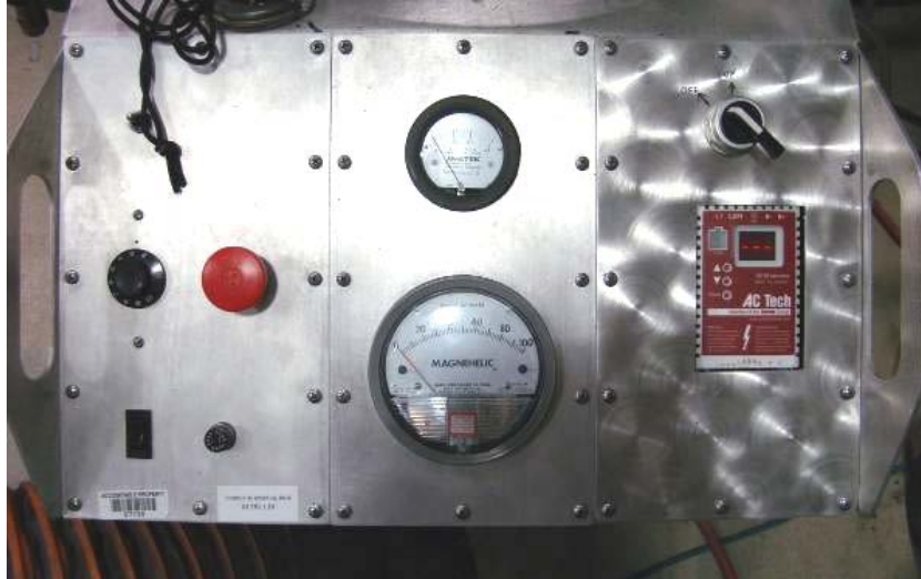
Figure 5.2. Control Panel with Gauges
