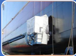
Paint/Solvent Operations Pintura /Solventes
